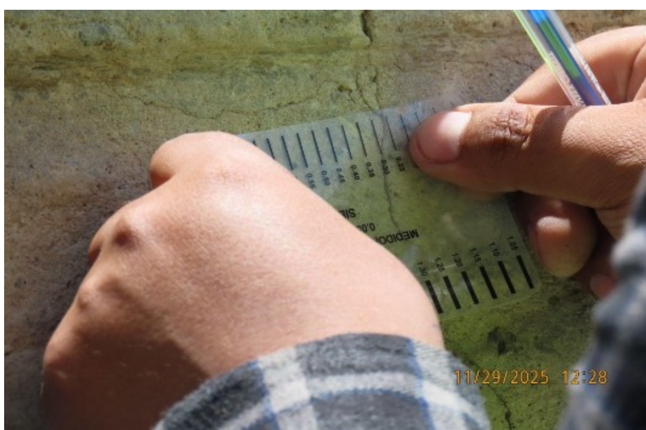
Figure 2: Manual crack measurement on bridge surface.
